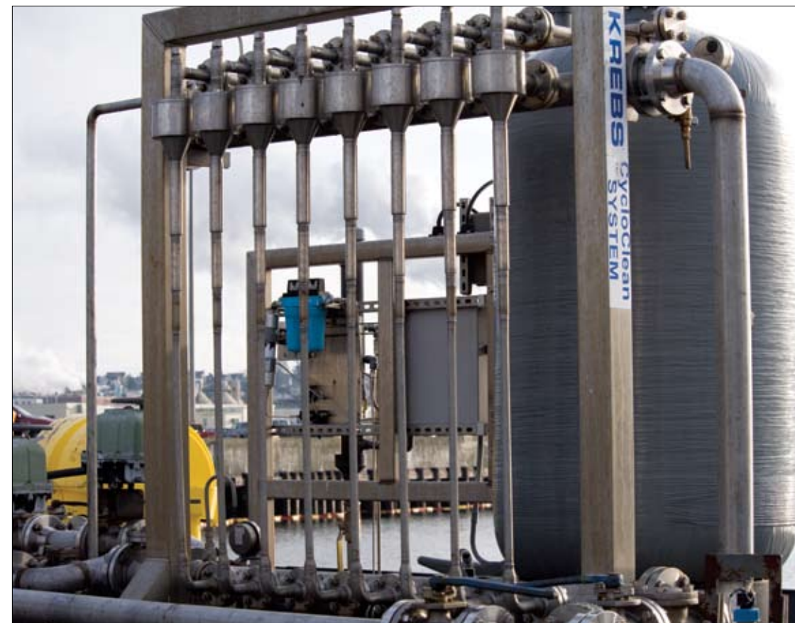
▲ The compwater treatment system sits atop a barge at Naval Station Everett.
